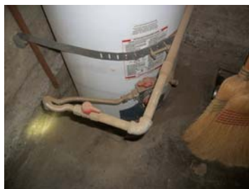
Both water heaters
